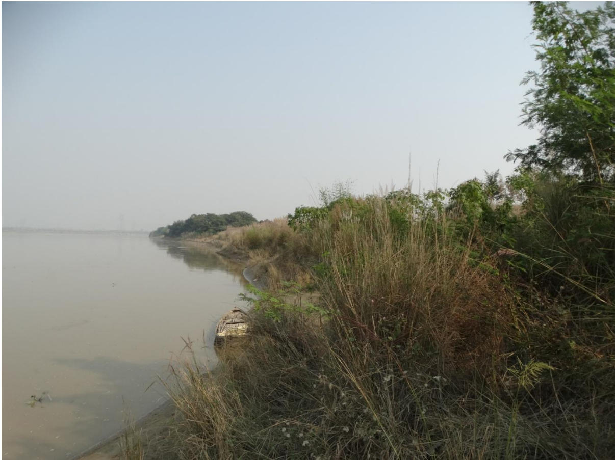
Image 50 : Stable Bank of River Ganga Near Bhueya Baba Temple Area [Right Bank]
